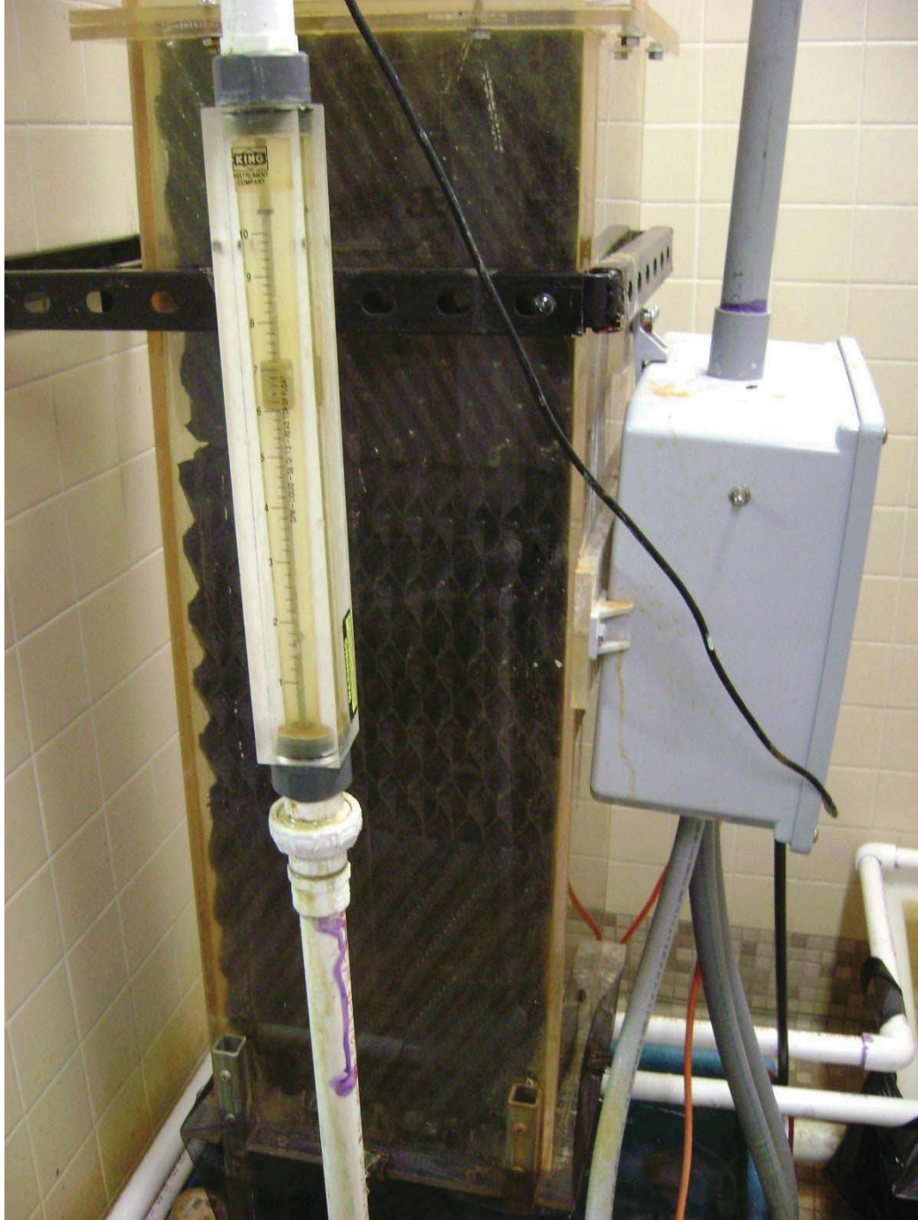
Figure G24 – T2 (Device) prior to UD trial.
