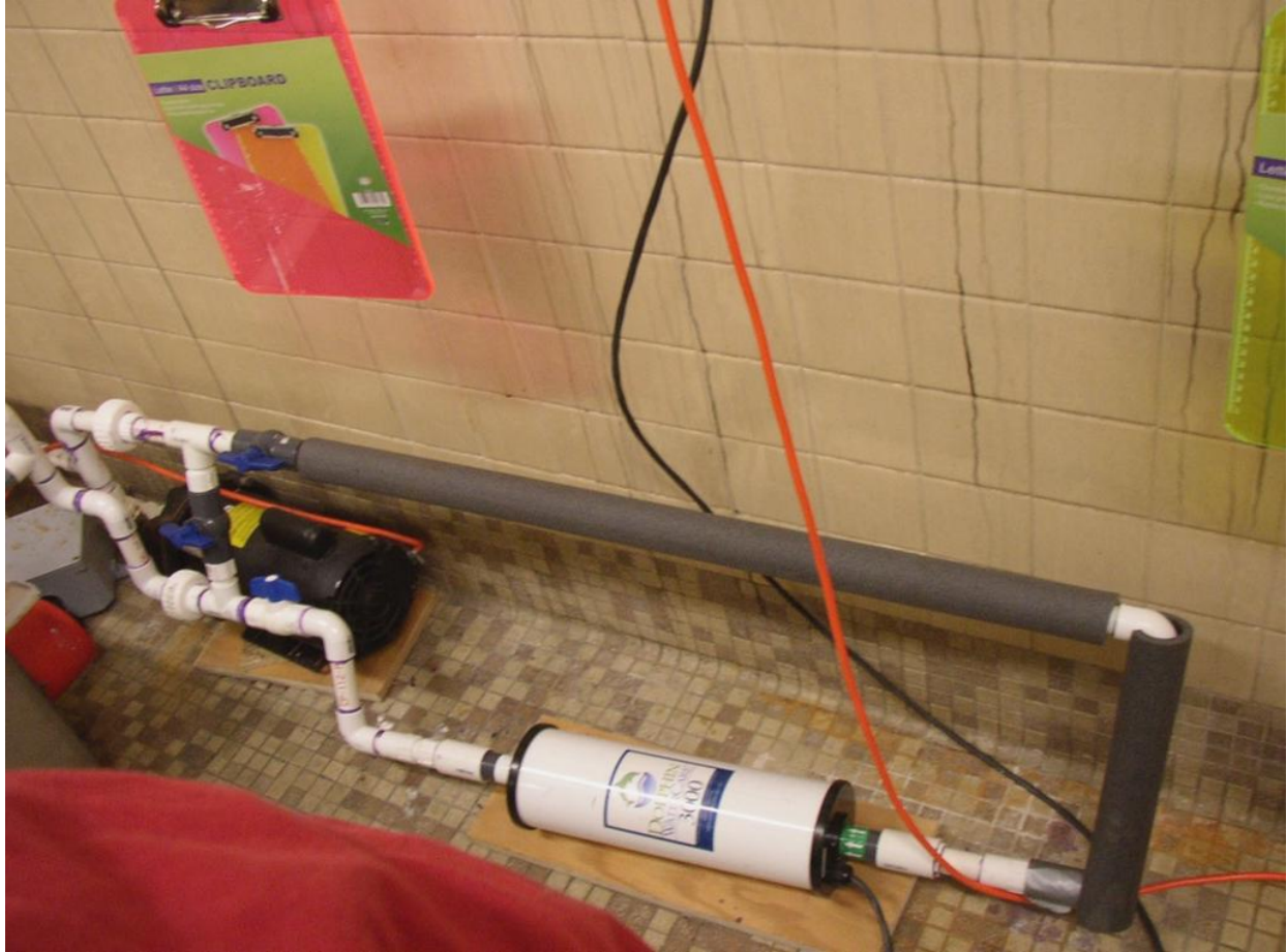
Figure D23 – PEFD installed on T2 (Device). Device placement is directly after pump and directly before entrance into heat bath.
